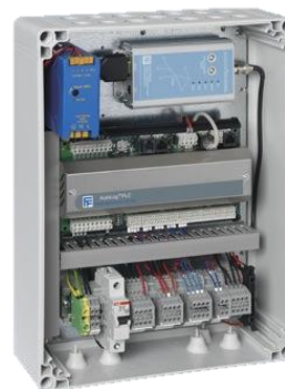
Remote Telemetry Unit - RTU
