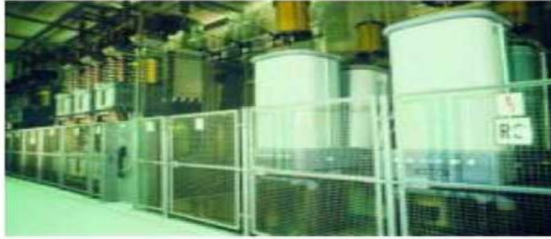
Figure 1: Mercury valves used in the Gotland HVDC transmission inaugurated in 1954
